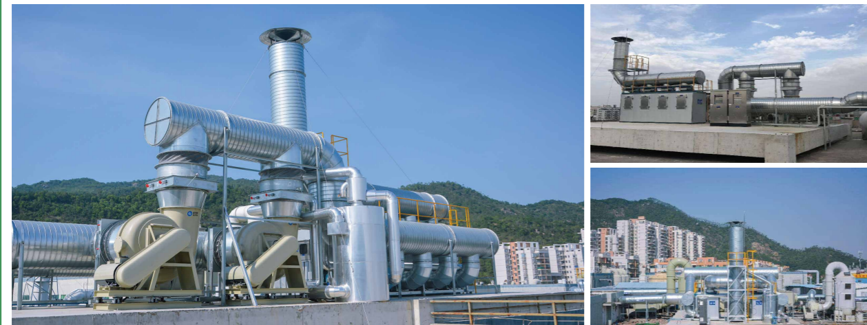
Exhaust gas end treatment device
