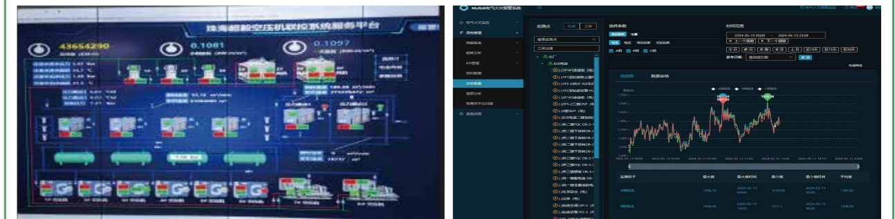
Compressed air system control platform
