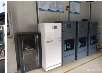
Industrial wastewater online monitoring device
